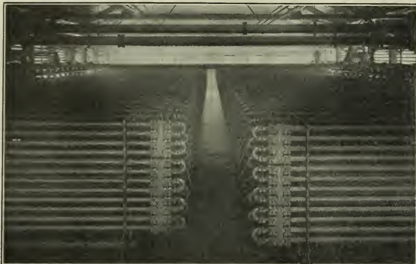
FIG. 3. AMMONIA CONDENSER ROOM
